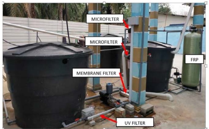
Figure 6: Filtration system for groundwater and rainwater
