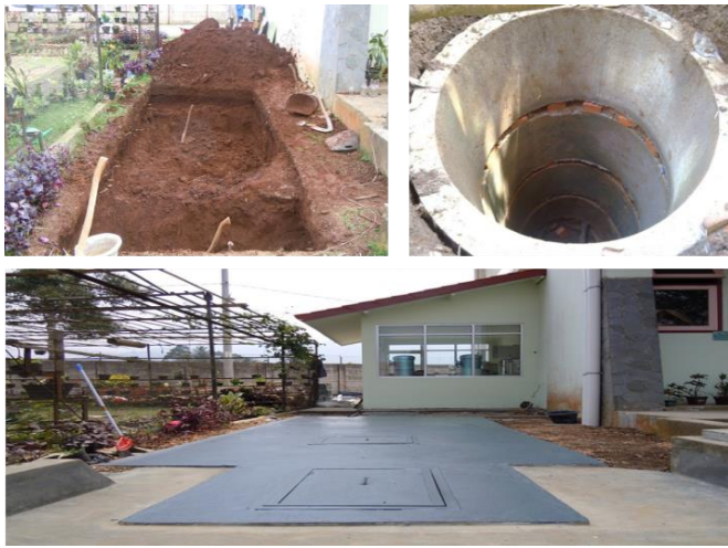
Figure 4: Construction of rainwater storage systems (RSS) and infiltration wells (IW) (Said, 2008; KELAIR, 2021)
